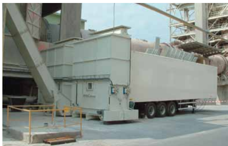
Fig. 4 Docking station with walking floor container
