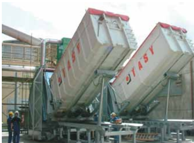
Fig. 5 Docking station with tipped container
